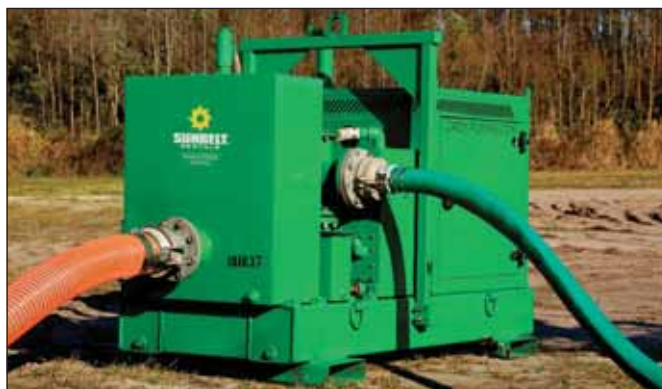
6" Sound-attenuated Diesel Wellpoint Pump
