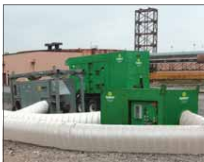
5,000 CFM Desiccant Dehumidifier, 320 kW Generator & 150 kW Heater
