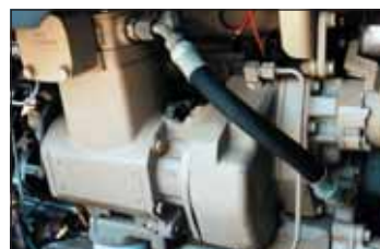
Direct-Drive Air Compressor
