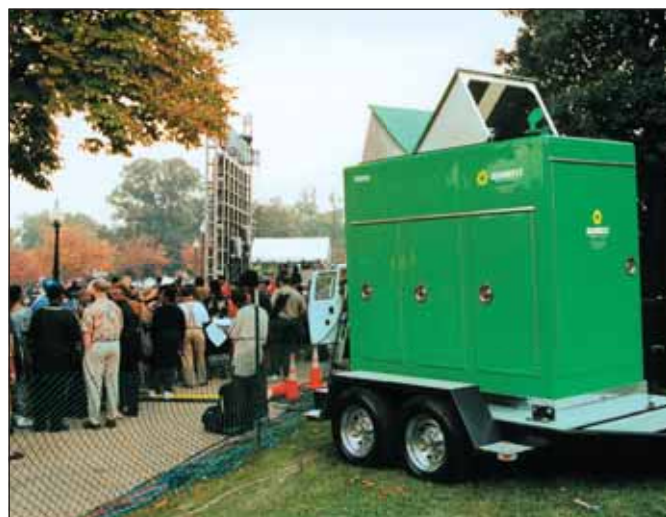
MQ 1,400 amp Movie Set Generator Powering video screens at an outdoor rally
