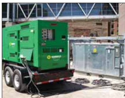
5,000 CFM Electric Desiccant Dehumidifier & 175 kW Generator
